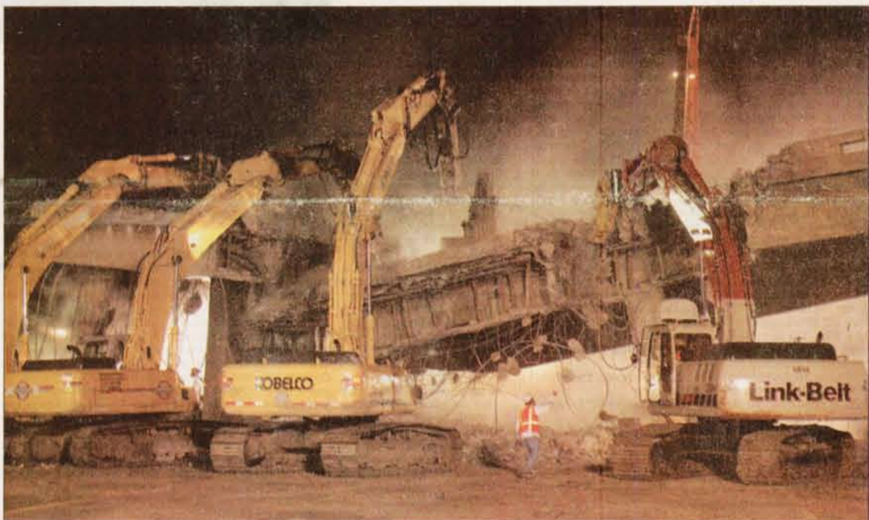
Workers and giant machines demolish the Layton Main Street bridge on Interstate 15 late Saturday night and early Sunday morning.
